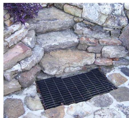
Drain inlet — set flush in a flagstone terrace
